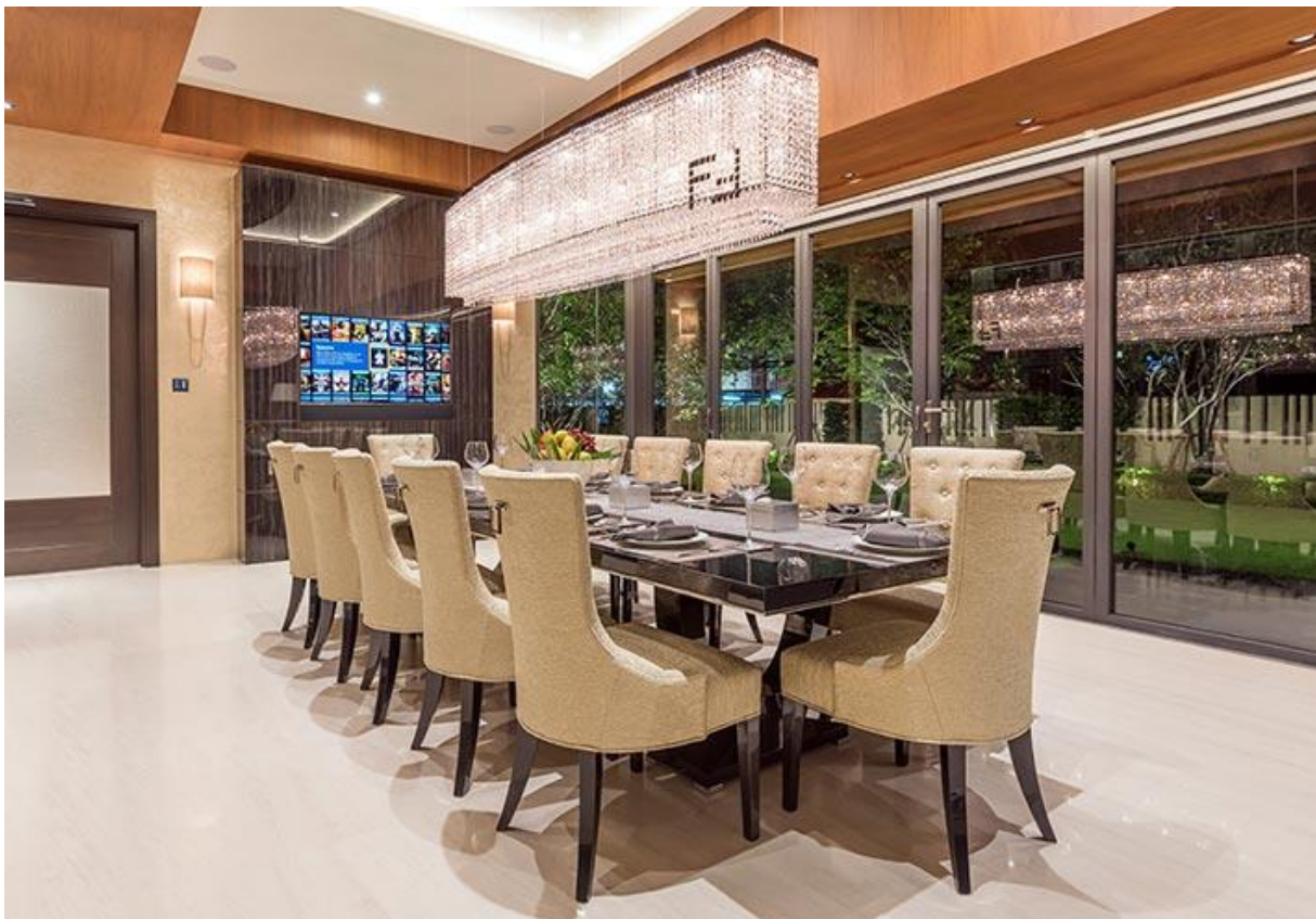
Future Automation SPS - Installed By NV Integration
